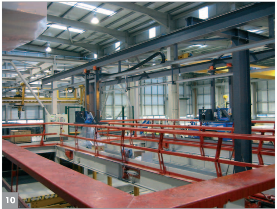
Mezzanine for manual shuttering
