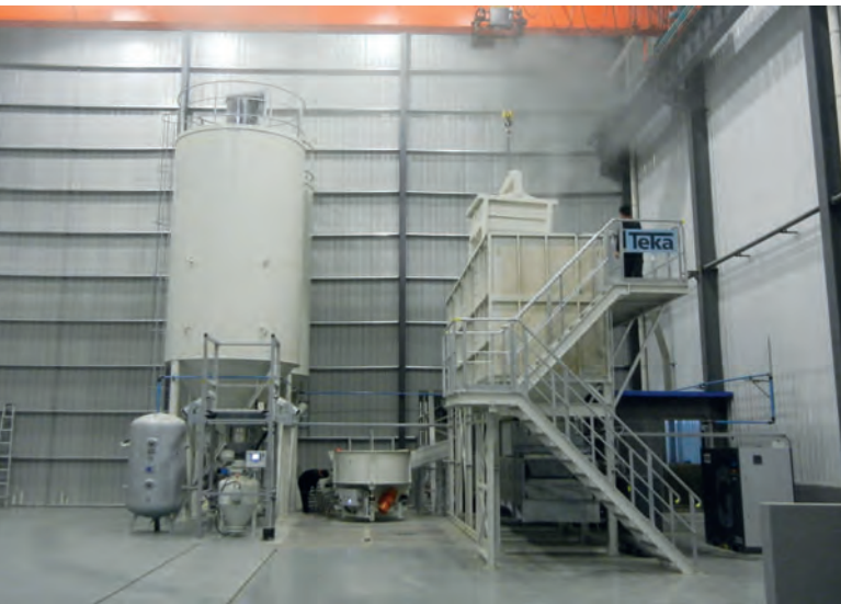
In-line silos and cement silos
